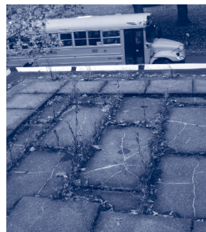
Portions of each school roof would be replaced. Many of these are in bad shape or starting to leak. This piece of the Middle School roof was last replaced in 1987.
