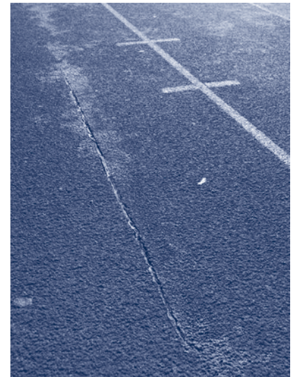
Cracks in the surface of the high school track have been repaired several times, but the entire track now needs to be rescaled to prevent these from growing and damaging the underlying structure of the track.
