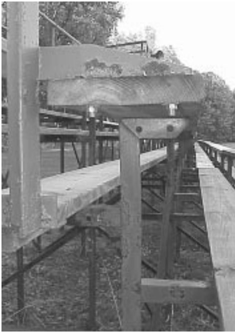
Maintenance staff have done their best to prolong the life of the High School football bleachers with paint and new wooden seats, but a outdoor metal structure dating from 1967 can't be expected to last much longer.
