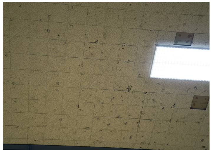
The high school's aged, disintegrating gym ceiling with missing and damaged tiles is in need of replacement.
