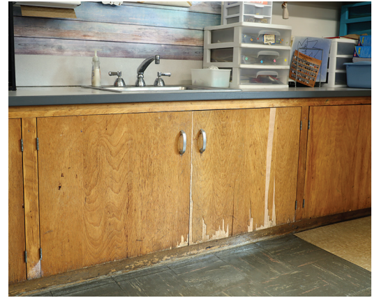
ABOVE Worn, splintered, and warped classroom cabinetry from the 50's and 60's and mismatched floor tiles can be found at all three elementary schools.
